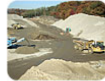
Very large stockpiles of the 2-inch crushed concrete, courtesy of Columbia Construction Company.
