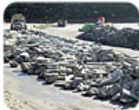
Granite curbing to be reused and asphalt to be crushed and reused, courtesy of Columbia Construction Company.
