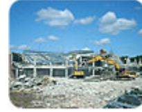
Existing concrete building being demolished with large excavators, courtesy of Columbia Construction Company.
