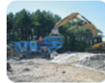
Of the 65,000 tons of material that comprised the actual weight of the demolished building, 61,000 tons of concrete and masonry block were crushed on site and used as structural fill.
